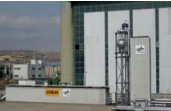
Demonstration combination storage system comprising concrete solid matter storage system (left) and latent heat storage system (right)
