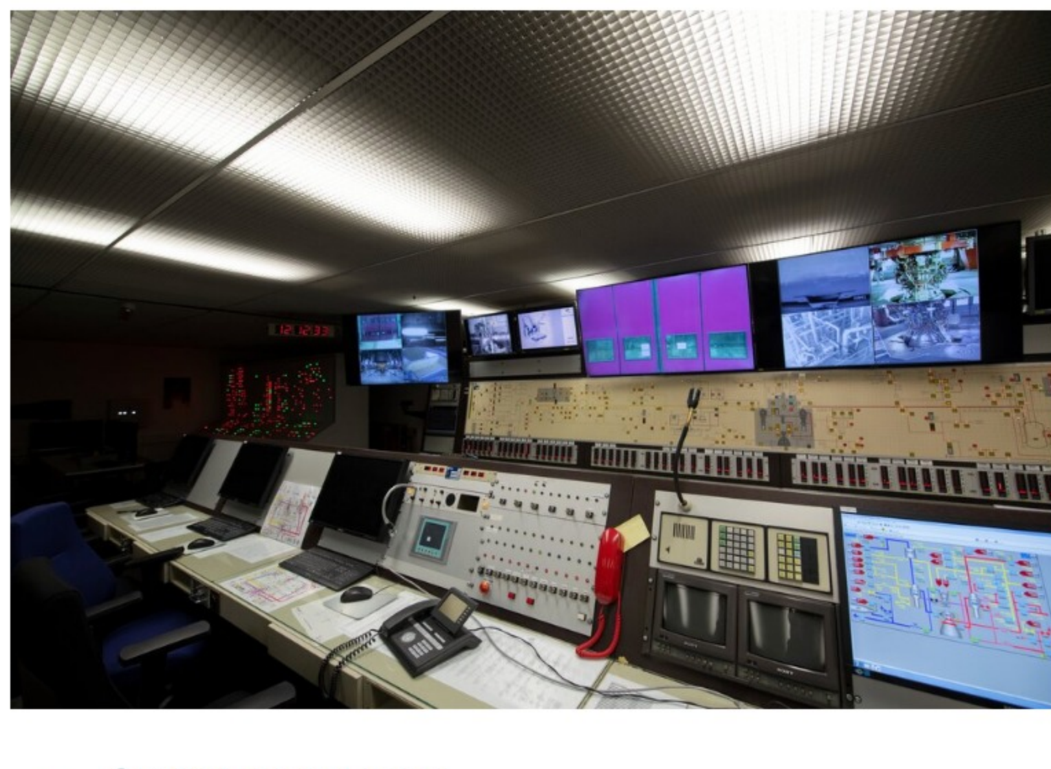
Central control room
