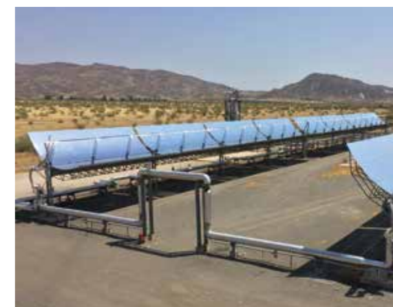
PROMETEO test facility at the Plataforma Solar de Almería
