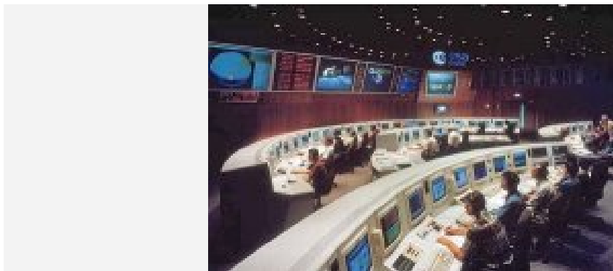
Main Control Room (MCR)
