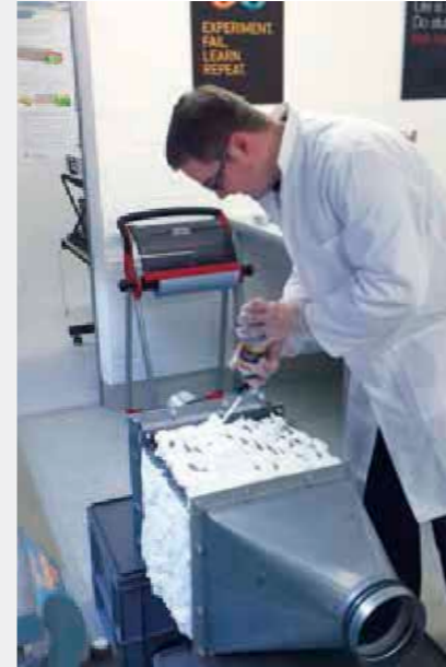
Paul Zabel inside the EDEN Laboratory, thermally insulating the air management cooling coil
